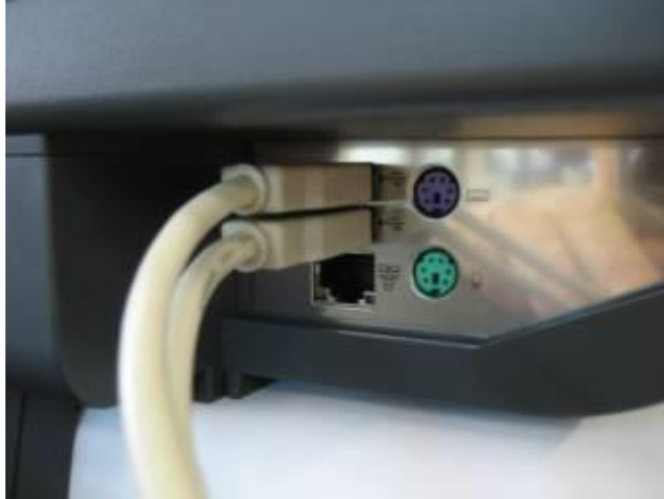
USB cables on bottom RHS of touch screen.
